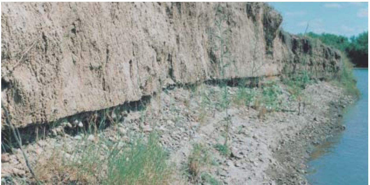
Fluvial scour at the high water toe of a bank. Photo Guy Roth.
