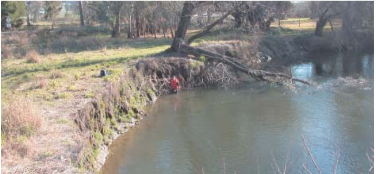
A typical abutment, but lone trees are eventually outflanked by erosion. Photo Ian Rutherford.
