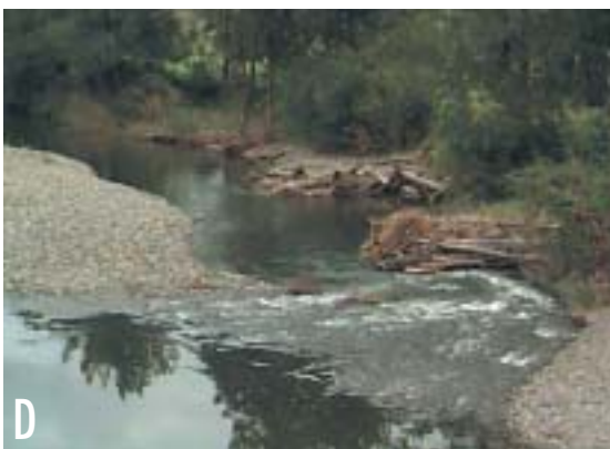
Figure 2: A. Upper section of Munni test reach at the commencement of construction of the upstream deflector jams. Note a 4 metre high actively eroding bank was located to the right of the tractor; B. The completion of construction; C. Same view in flood (270 m 3 sec -1 , 7/05/01) at about 1 metre below peak stage; D. Following the second major flood since construction — note the aggraded bar upstream of first structure and the increased scour around the two structures. The riffle crest in the foreground was raised as a result of backwater effects associated with the structures. Photos Andrew Brooks.
