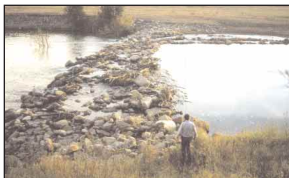
Figure 45. A mangfall sill with central fishway (photo by John Harris).
