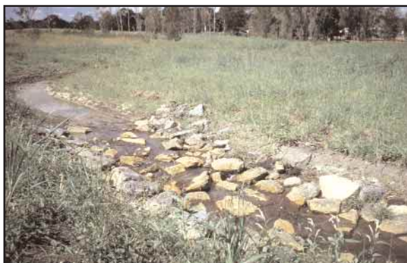
Figure 4. Artificial riffles created in a re-meandered, cohesive bed stream in Brisbane. The riffles act as low dams, effectively reducing the scour velocity on the cohesive bed material.
