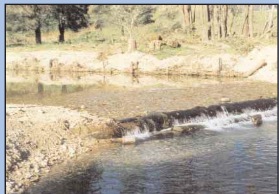
Figure 11. A freshly constructed straight, stepped log sill on Taylors Arm, northern New South Wales (photo by Allan Raine).
