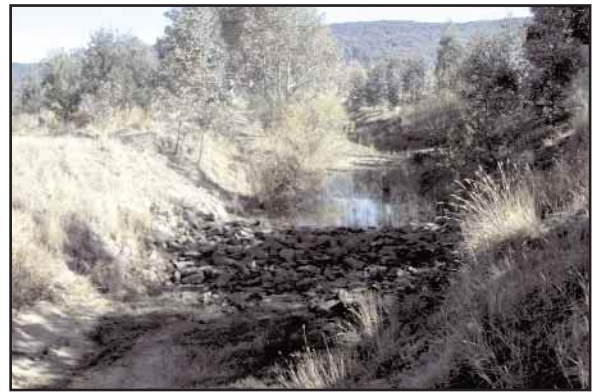
Figure 31. These pools in Reedy Creek have been created by the construction of rock chutes.
