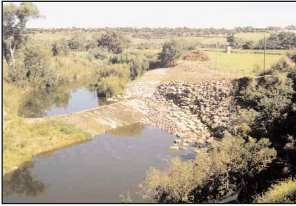
Figure 49. An off-stream rock-ramp fishway constructed by Melbourne Water around a weir on the Maribyrnong River, Melbourne. This is a similar design to the bypass structure on the Barwon River.
